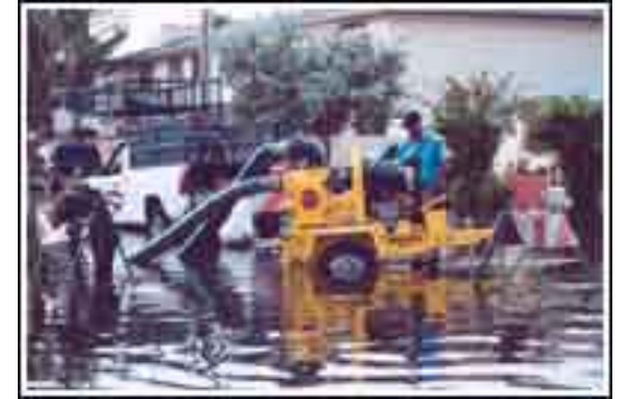
Flood, Water Main Miami, FL
