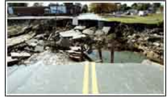
Washed out bridge, Tobarro, NC
