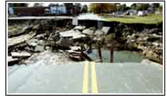
Washed out bridge, Tobarro, NC
