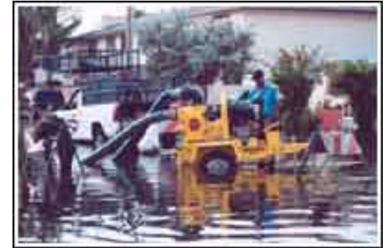
Flood, Water Main Miami, FL
